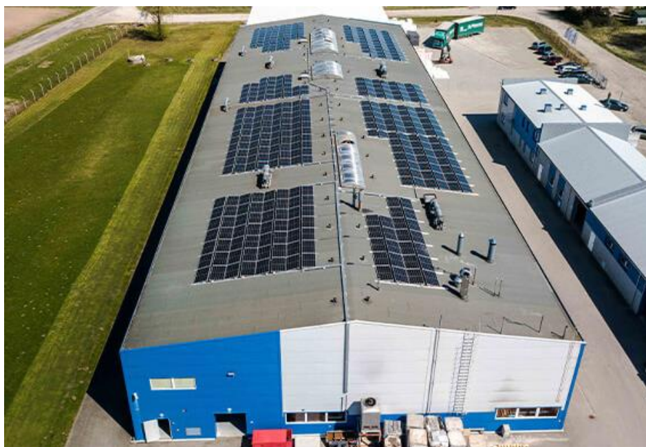
Kauno šilas UAB solar panel system on the roof of manufacturing plant
